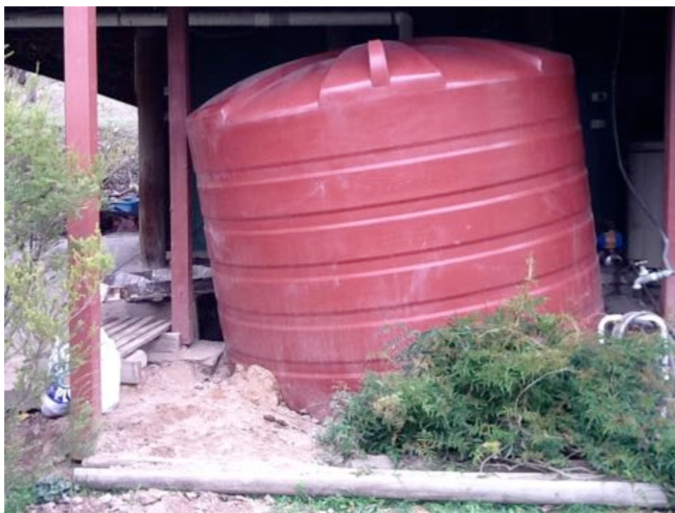
Figure 6. Wombat burrow under the water tank at Micalong Creek. Image courtesy of Affrica Taylor
